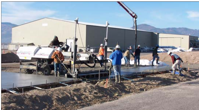
Pouring of concrete pads is nearly complete at GA hangar construction site, Oct 2008.
