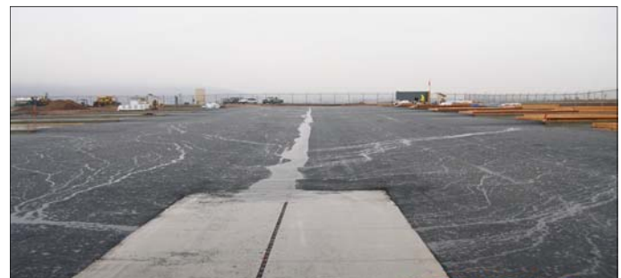
Completed taxiway/apron at the construction site for the new GA hangars, showing effectiveness of drainage. Oct 2008.
