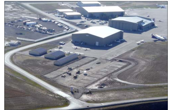
↑ Construction site of new GA hangars, near Northstar, Sept 08. Mike Kustudia photo
